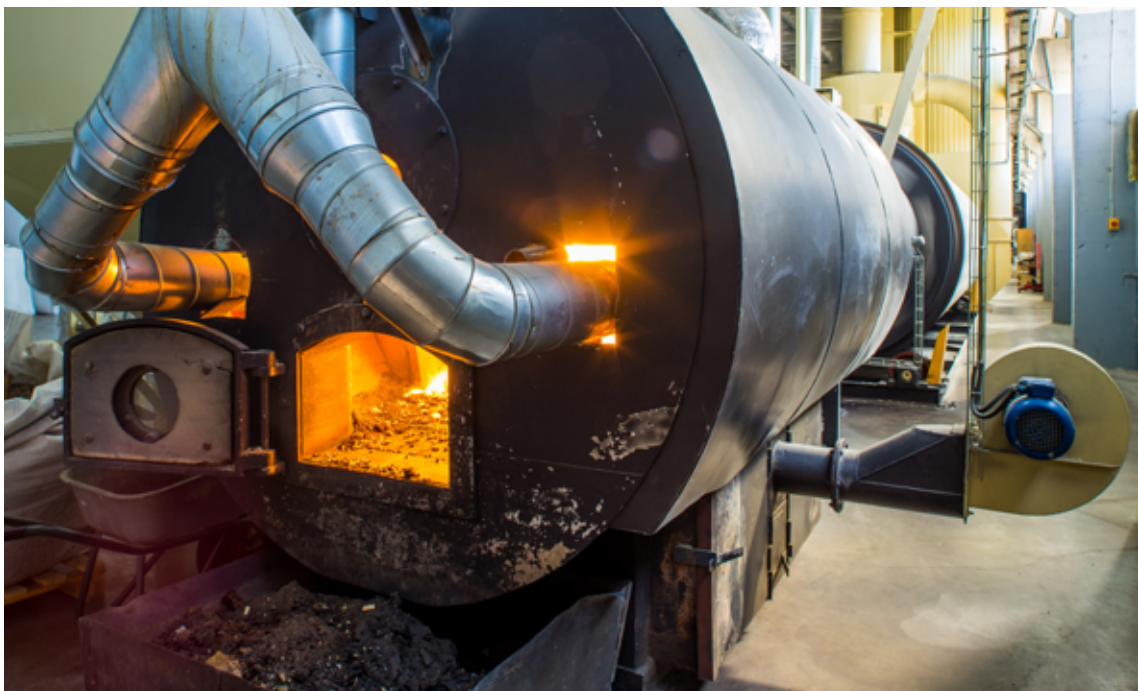
Wooden pellets boiler.
