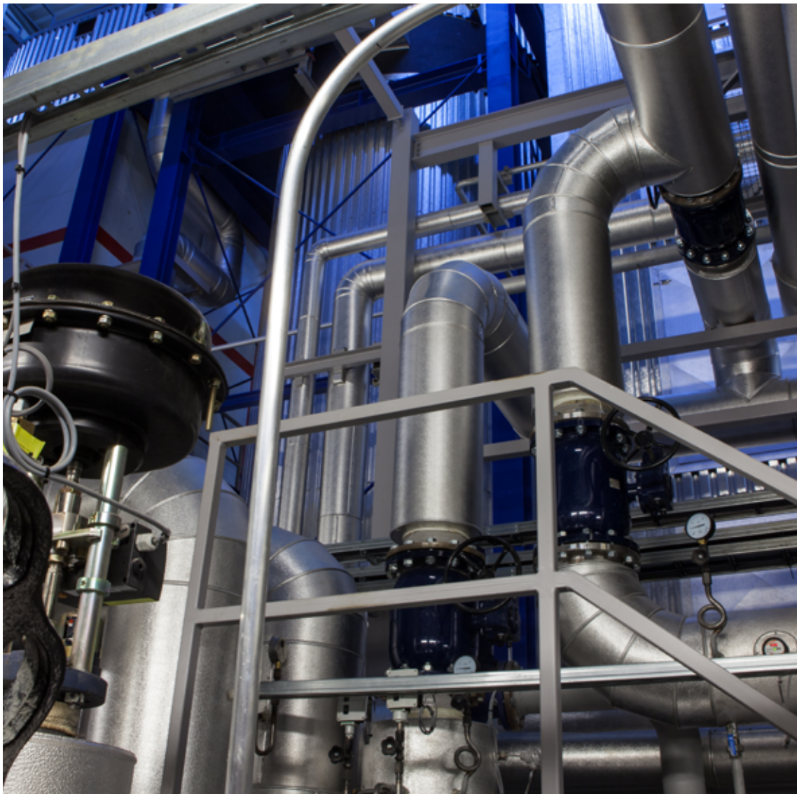
Modern biomass co-generation power plant.
